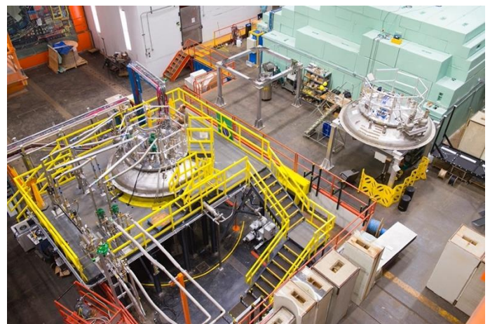
Colossus: SQMS is developing the world's largest and highest cooling power dilution fridge, capitalizing upon Fermilab's unique facilities and expertise in cryogenics.
